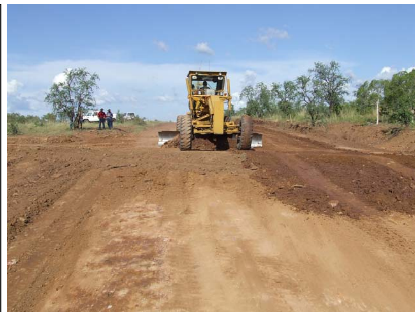
The final touch up on a newly installed diversion bank at Carlton Hill Station.
