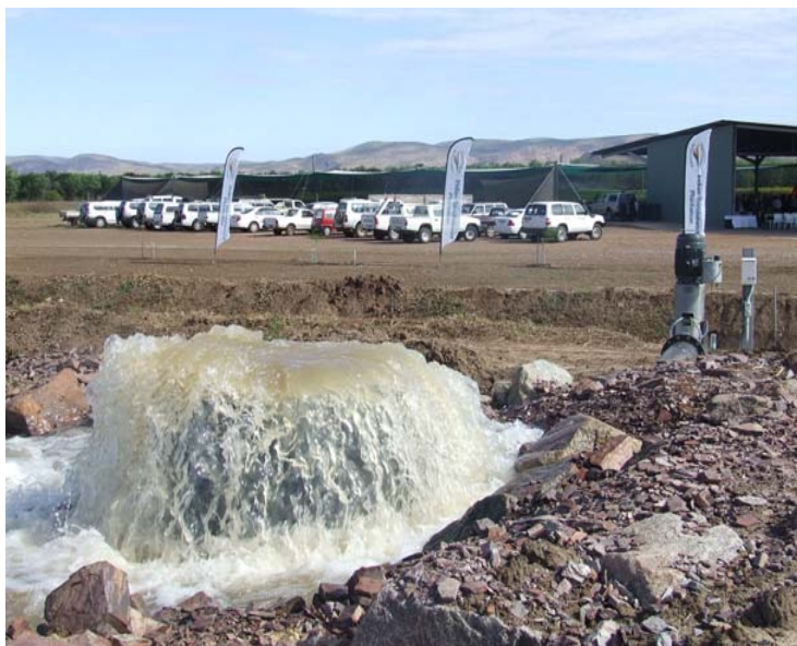
The pump lifting water up into the channel for re-use is switched on.
